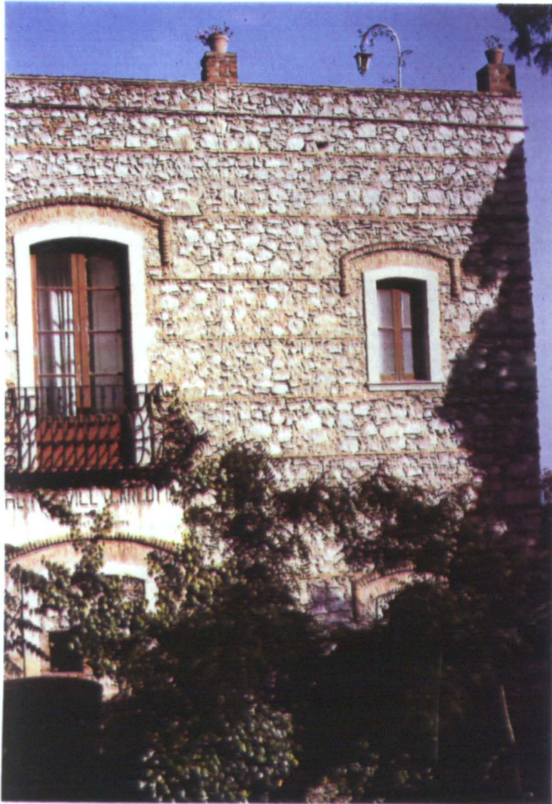
6.42 Rear of the Hotel Bristol (now Villa Carlotta ), Taormina, in 1992. The brick-levelled roughstone courses and relieving arches over every aperture are clearly visible.
