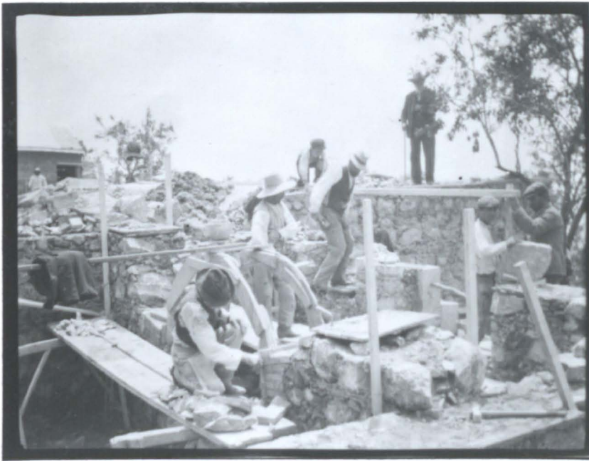
6.47 Erecting the centering for one of the arches under the supervision of Don Nino Siligato.
