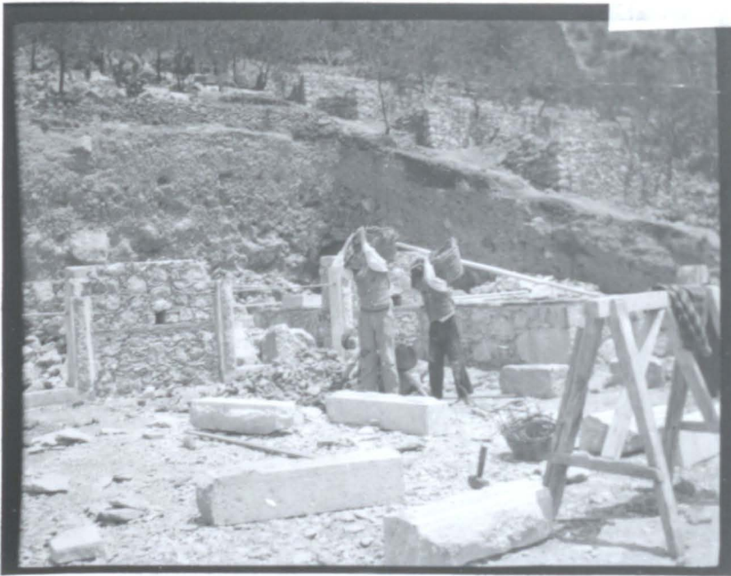
6.48 The stone lintels were dressed on the site, which was cut into the almond and olive terraces.
