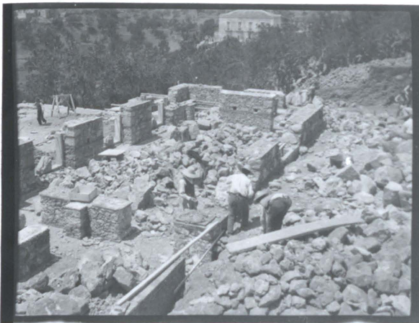
6.49 Casa Cuseni at the first lift of wall construction. Beyond is the Villa Strazzeri (R.H.K. photos).
