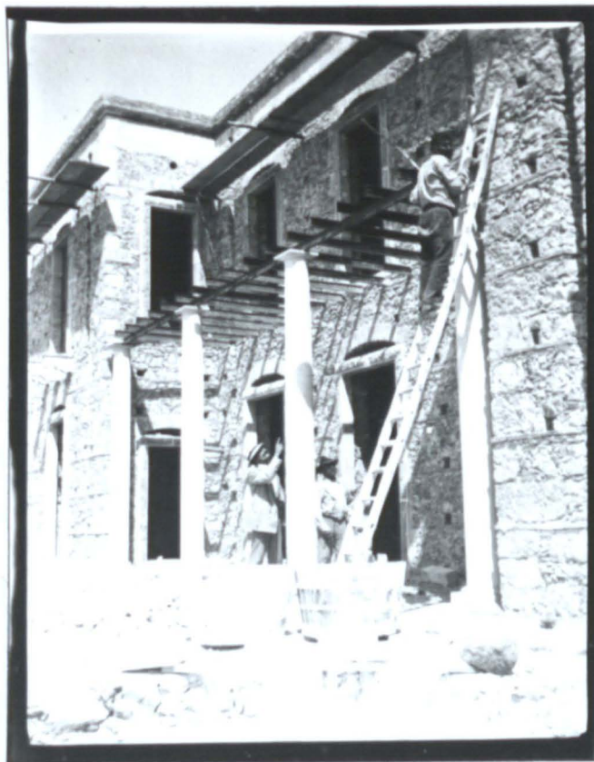
6.51 The front of Casa Cuseni . Note the relieving arches with lintels in position, the I beams over the loggia , the coursing layers and pudlocks, and the first application of stucco below the cornice.
